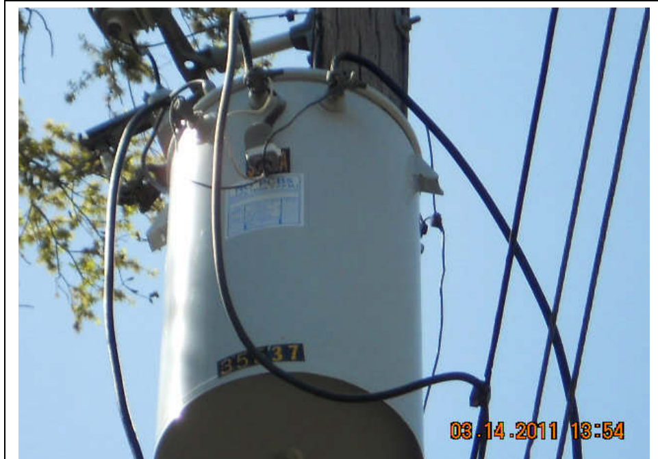
Photograph 5: Pole-mounted transformer with "non-PCB" label.
