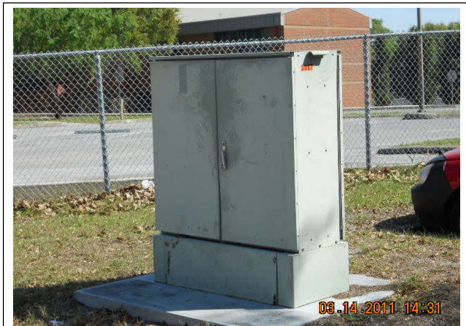
Photograph 6: View of pad-mounted transformer located south of Central office.
