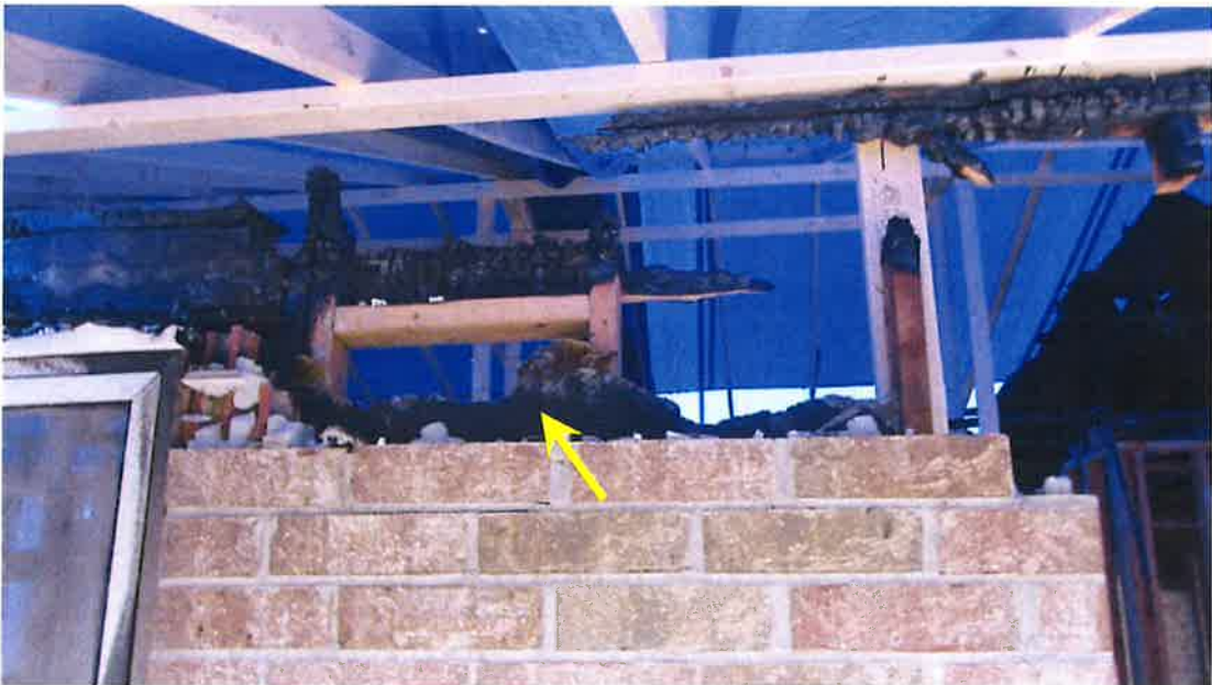
Photograph 62) – View looking east at the rear exterior brick cladding at Unit #21. Repair of missing brick required.
