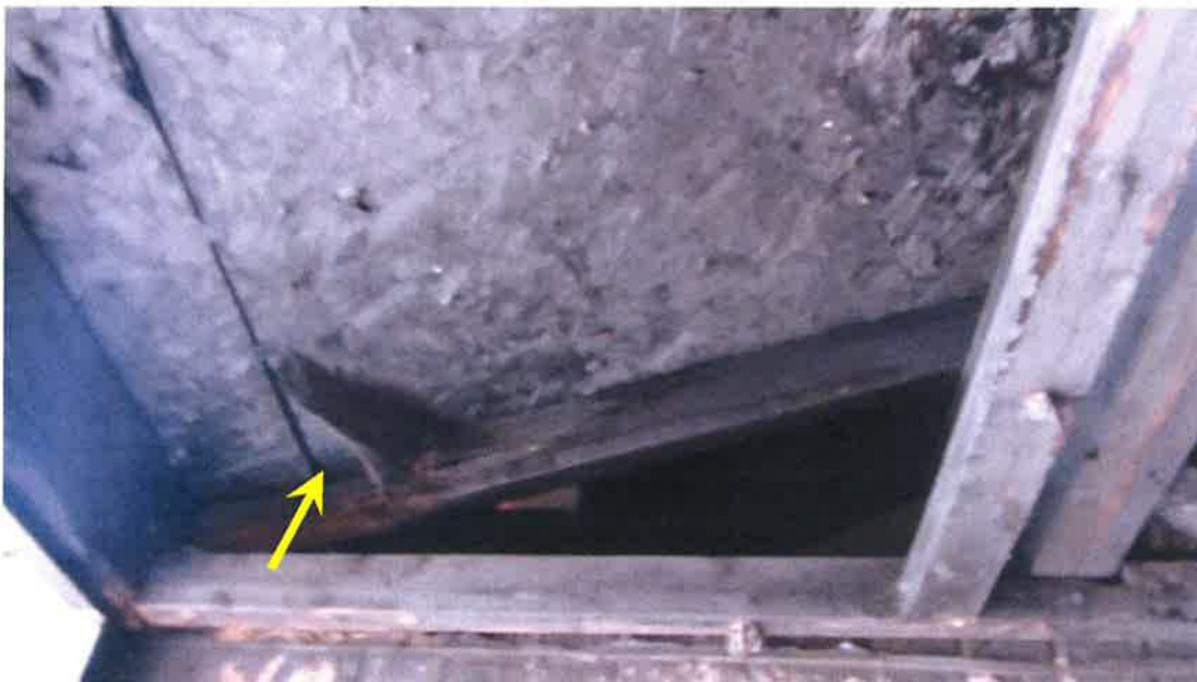
Photograph 34) – Close-up view of OSB sheathing and wood roof and ceiling framing above the front entry foyer of Unit #20 requiring replacement.
