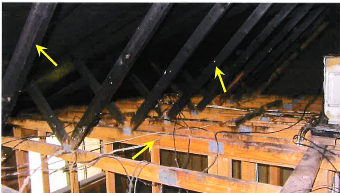
Photograph 26) – View looking southeast at pre-engineered Trusses 1 through 7 above the southern portion of Unit #20. Arrows indicate fire-related effects from smoke.
