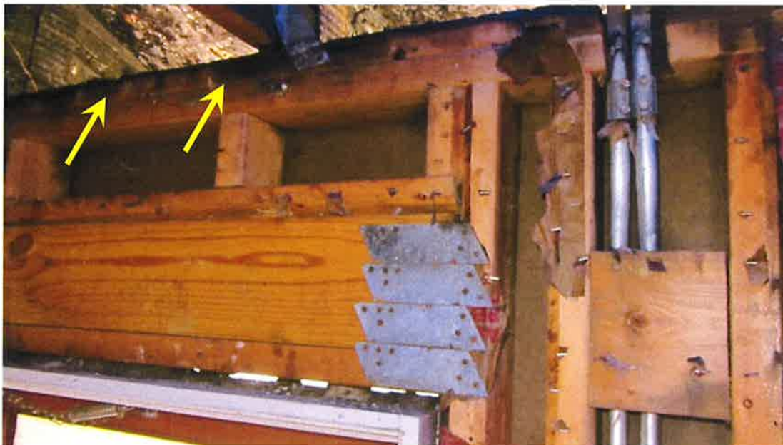
Photograph 40) – Interior view at a header and exterior load-bearing wall framing at the front elevation. Arrows indicate fire-related effects from smoke at the top plate of the wall.
