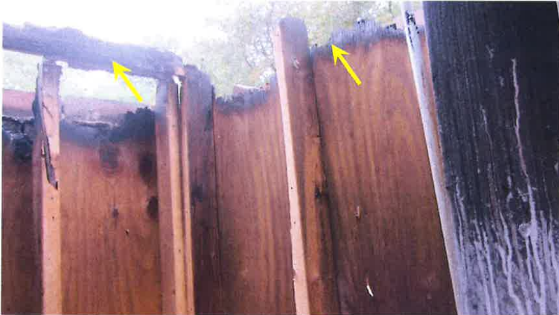
Photograph 53) – View looking southwest at the exterior utility closet at the rear of Unit #22. Arrows indicate fire-related damage to the upper portion of the wall framing system requiring replacement.
