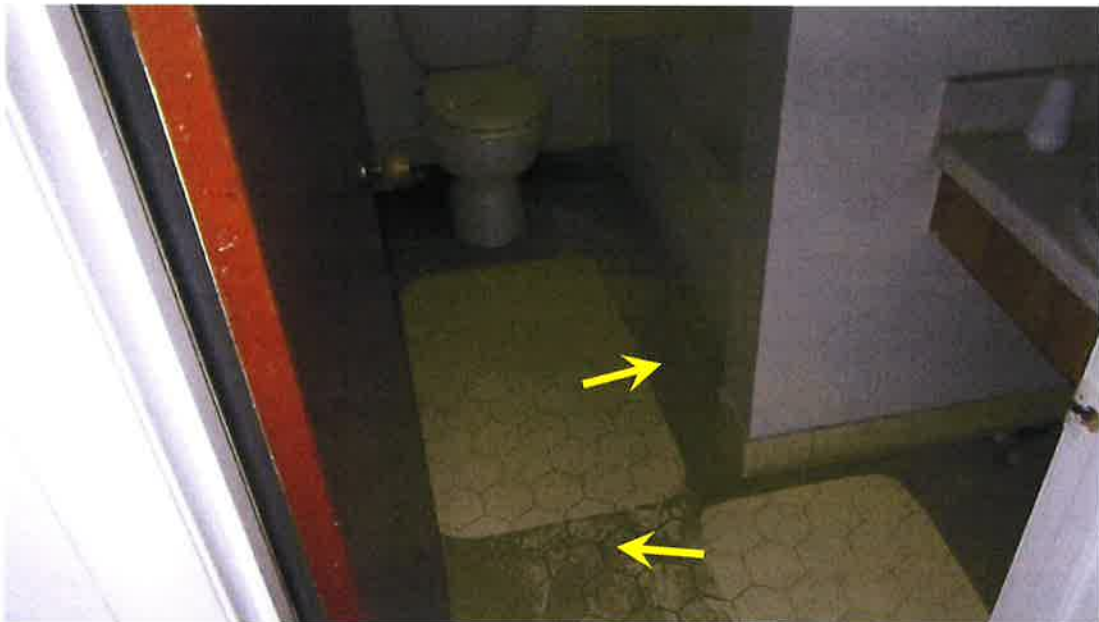
Photograph 12) – View looking west into the bathroom of Unit #19. Arrows indicate fire-related effects from smoke.
