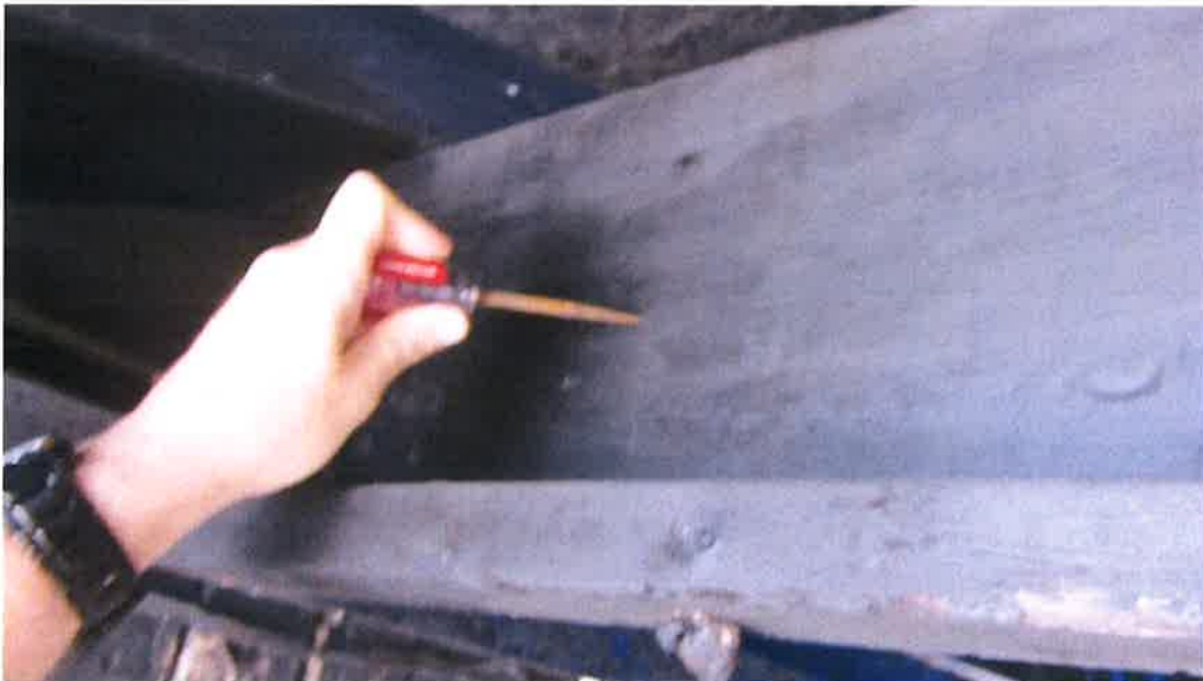
Photograph 36) – Close-up view of the east face of the double 2x12 wood header beam at the front entry foyer of Unit #20 requiring repair.
