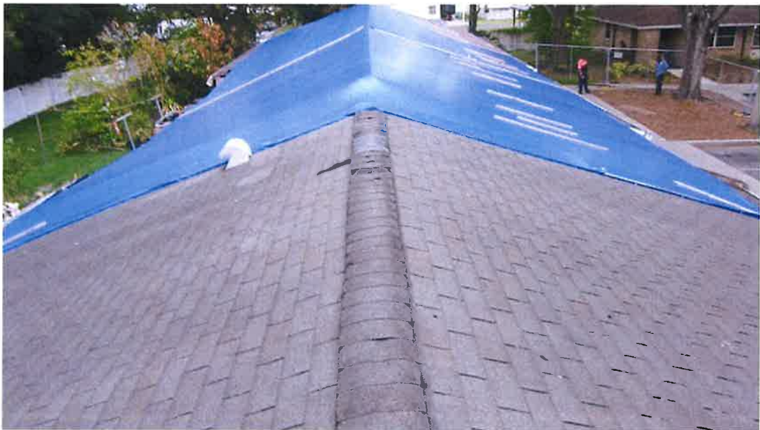
Photograph 20) – Roof overview looking north along the ridge of the remaining roof above the southern portion of Unit #20.
