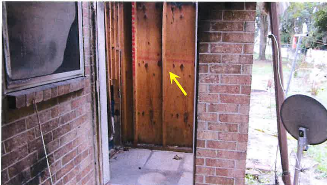
Photograph 52) – View looking south at the exterior utility closet at the rear of Unit #22. Arrows indicate the lower portion of the wall framing system with no fire-related effects or damage.
