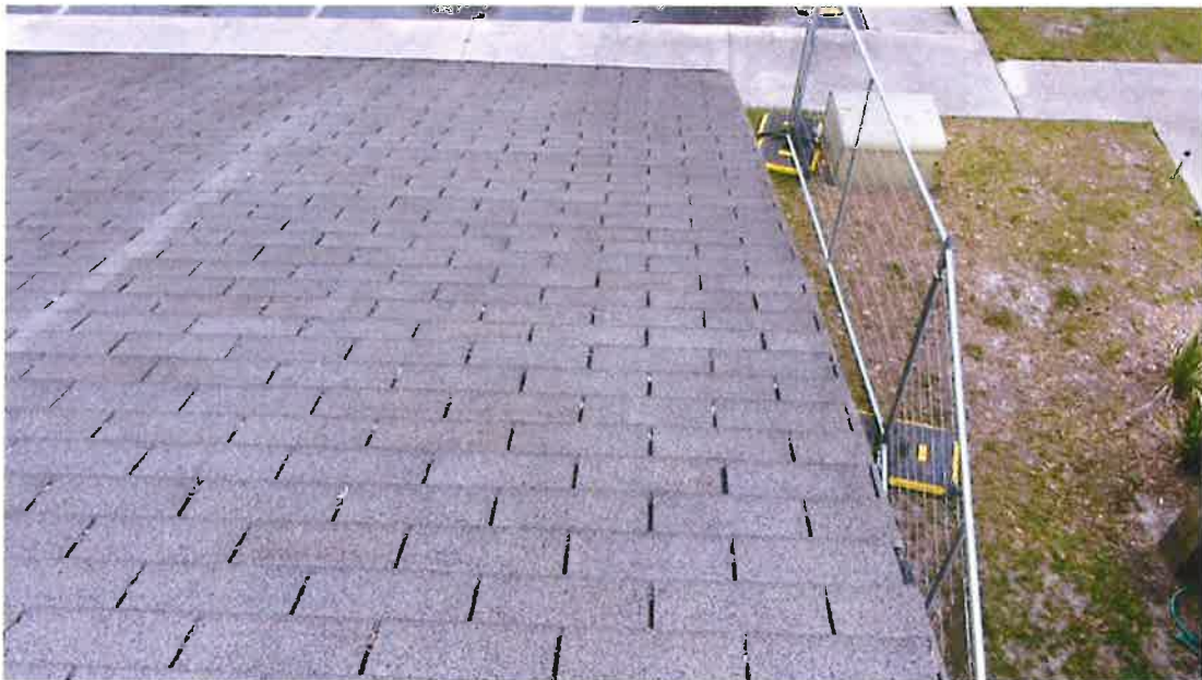
Photograph 16) – Roof overview looking east along the rake at the south gable end above Unit #19.
