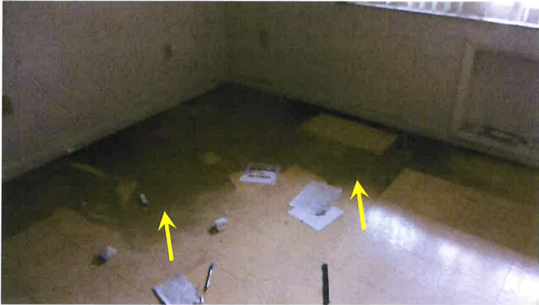
Photograph 11) – View looking northeast into the bedroom at the front of Unit #19. Arrows indicate fire-related effects from smoke.
