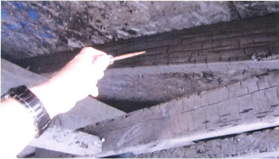
Photograph 35) – Close-up view of OSB sheathing and wood roof and ceiling framing above the front entry foyer of Unit #20 requiring replacement.
