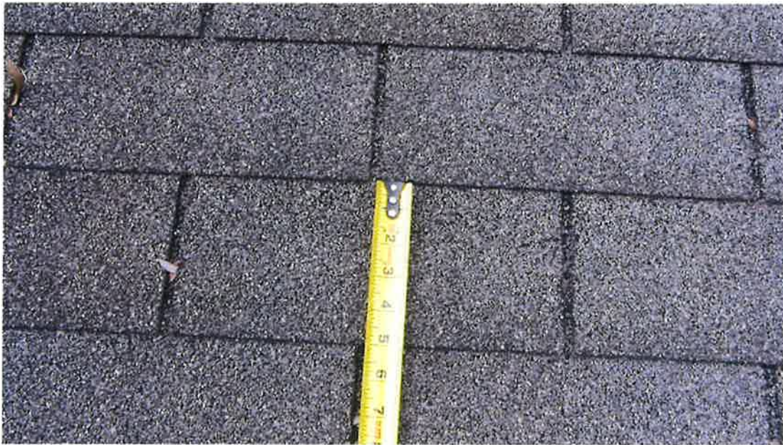
Photograph 23) – Close-up view of the three-tab, asphalt shingles above Unit #20 with an approximate exposure of 5 inches tall by 36 inches wide.
