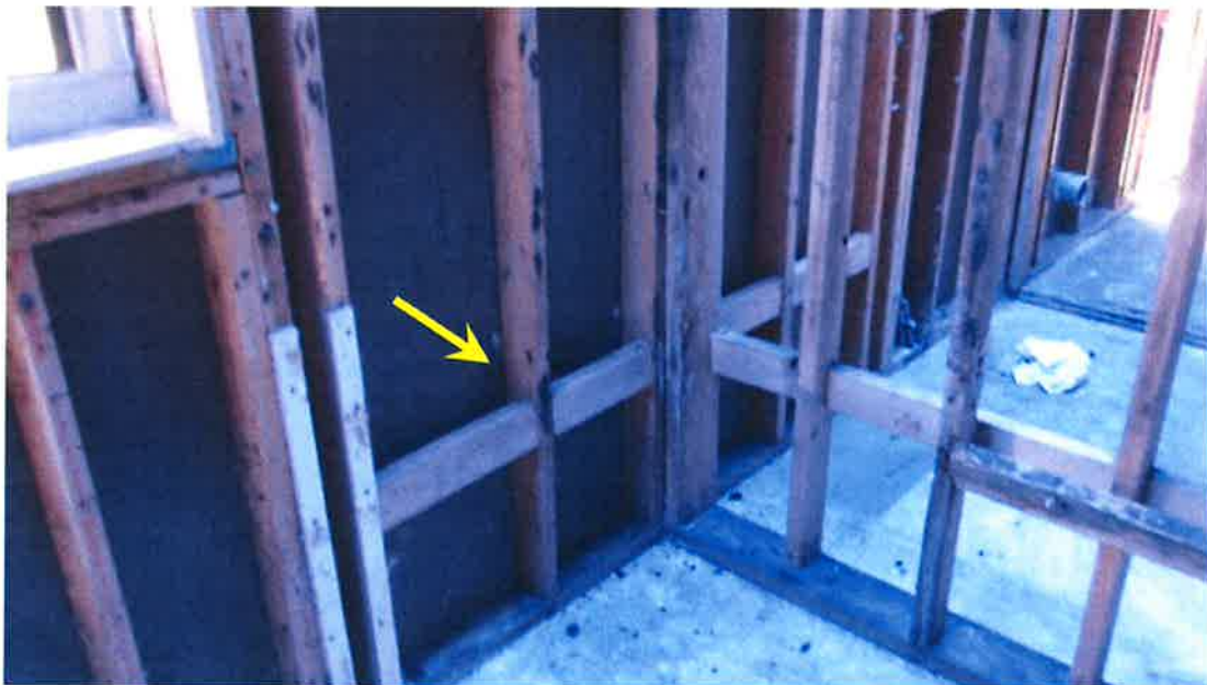
Photograph 46) – Interior view of the lower portion of the rear exterior load-bearing wall framing at Unit #22. No repairs required.
