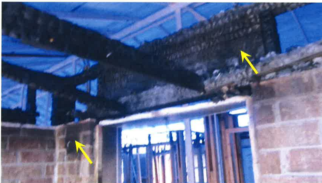
Photograph 60) – View of the exterior brick cladding at the front entry foyer of Unit #22. Fire-related effects from smoke shown with arrows.
