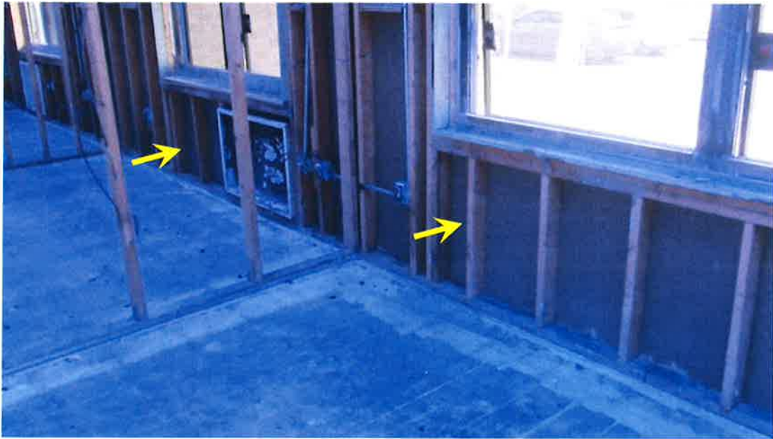
Photograph 45) – Interior view of the lower portion of the front exterior load-bearing wall framing at Unit #21 and #22. No repairs required.
