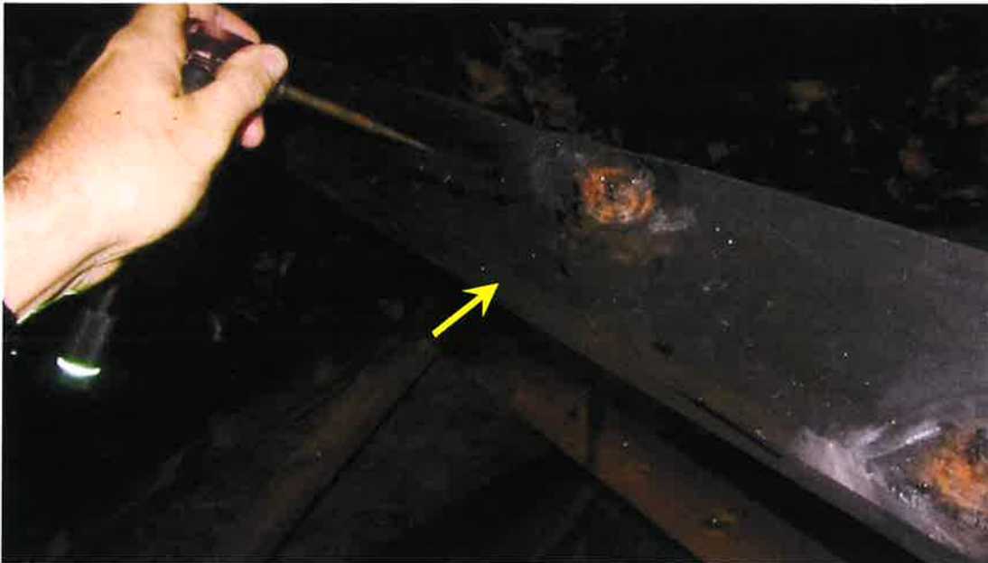
Photograph 29) – Close-up view of a pre-engineered wood truss above Unit #20 with fire-related effects from smoke. No structural damage was found when probed with the awl.
