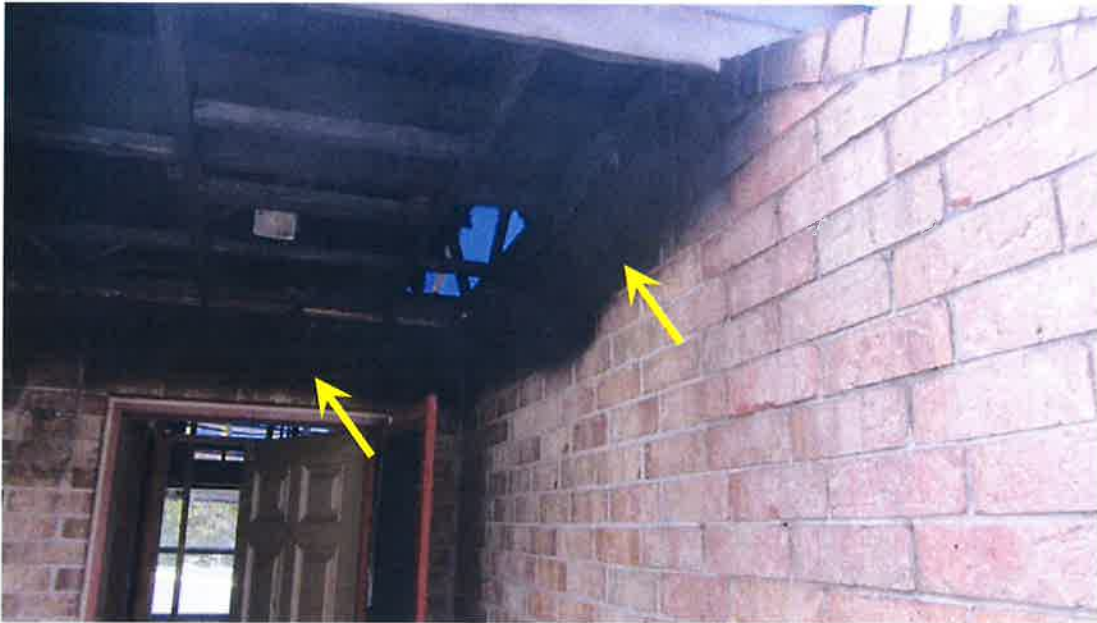
Photograph 57) – View of the exterior brick cladding at the front entry foyer of Unit #21. Fire-related effects from smoke shown with arrows.
