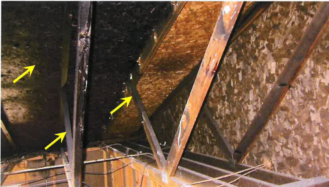
Photograph 25) – View looking east at the wood roof framing system above the southern portion of Unit #20. Arrows indicate fire-related effects from smoke.
