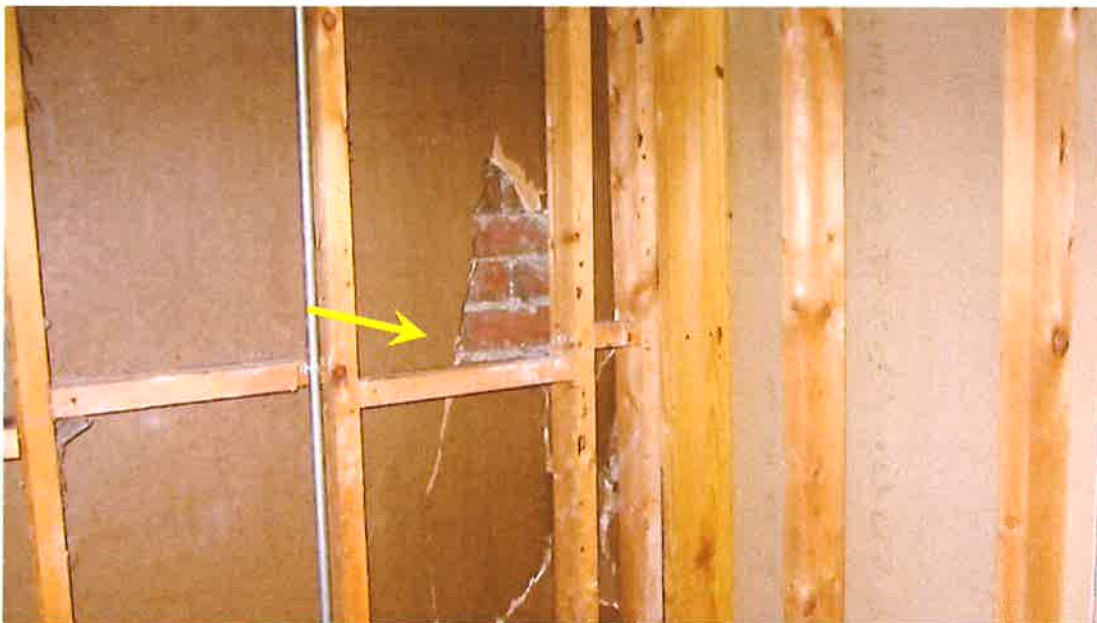
Photograph 38) – Interior view of the exterior load-bearing walls at the southeast corner of Unit #20. A hole in the sheathing requiring repair is visible with the backside of the exterior brick cladding visible.
