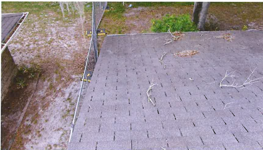
Photograph 18) – Roof overview looking west along the rake at the south gable end above Unit #19.
