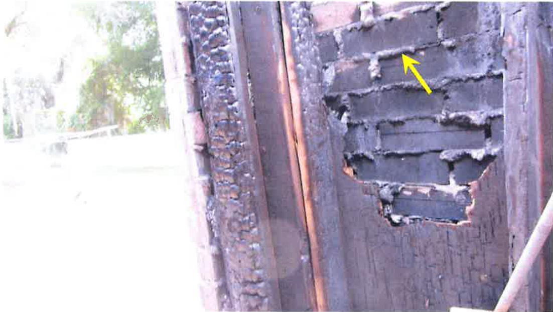
Photograph 61) – Close-up view of the rear exterior utility closet at Unit #21. Arrow indicates backside of brick cladding with fire-related effects. No repair required.
