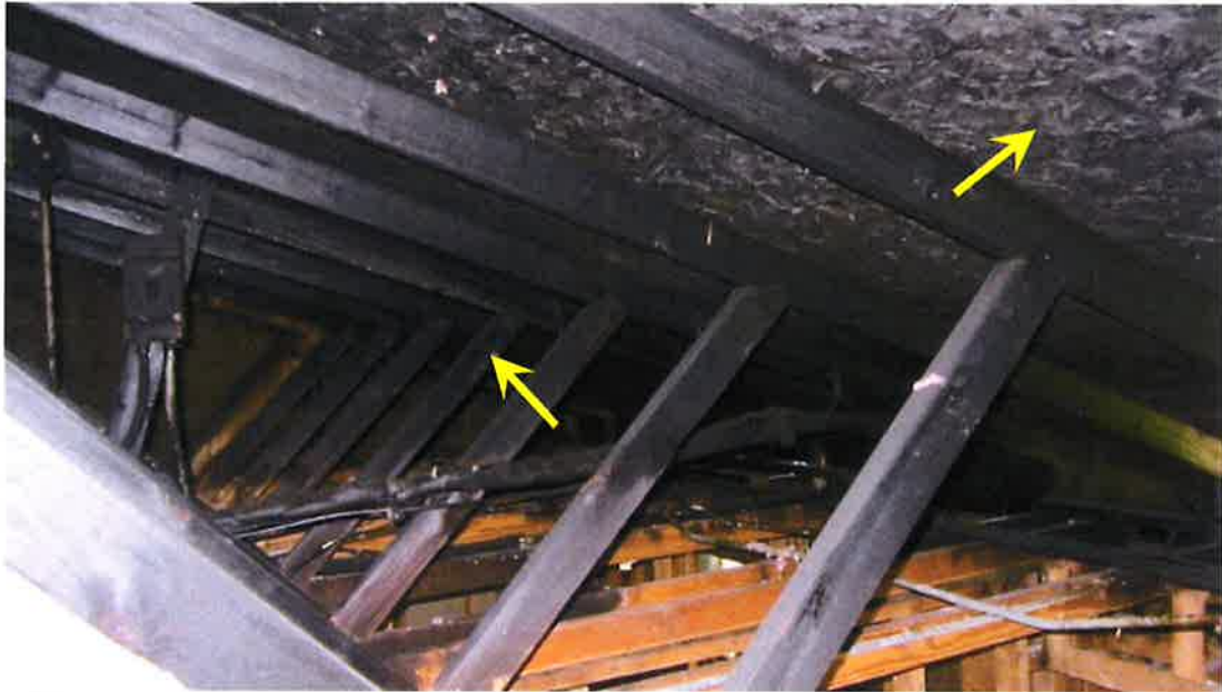
Photograph 27) – View looking southwest at pre-engineered Trusses 1 through 7 above the southern portion of Unit #20. Arrows indicate fire-related effects from smoke.
