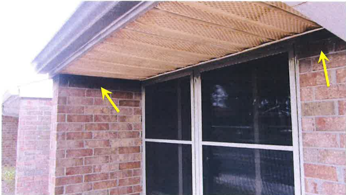
Photograph 56) – View of the exterior brick cladding. Fire-related effects from smoke shown with arrows.
