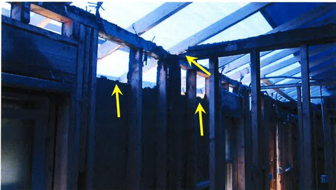
Photograph 42) – Interior view looking northwest at interior partition wall (right) and the rear exterior load-bearing wall of Unit #21. Arrows indicate upper portion of rear load-bearing wall framing system and interior partition requiring replacement.
