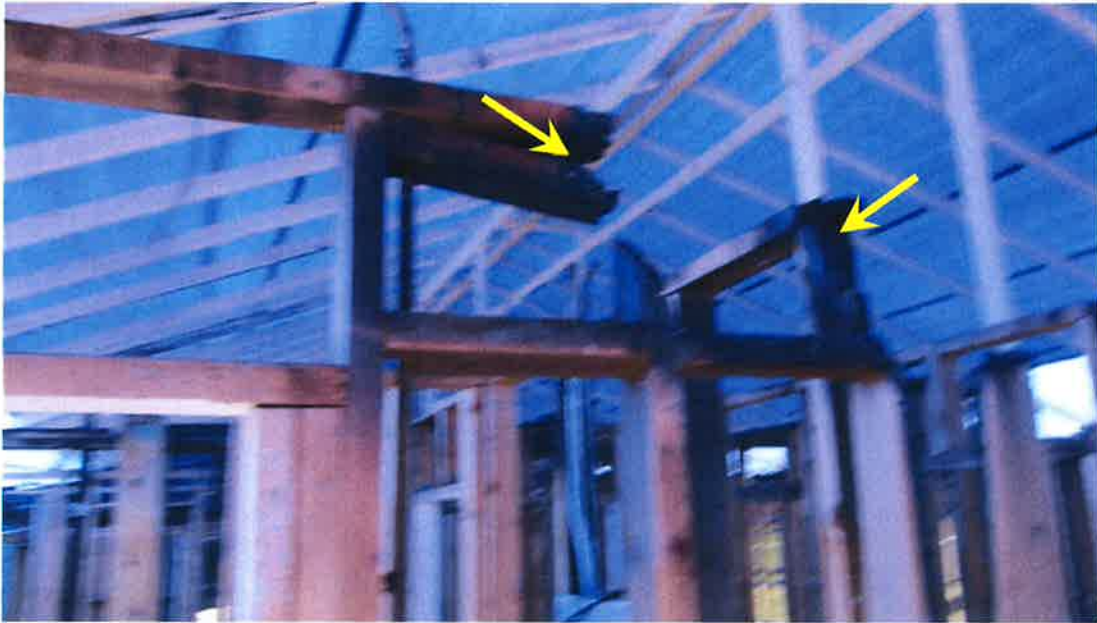
Photograph 47) – View of the upper portion of an interior partition wall in Unit #21 with fire-related damage requiring replacement.
