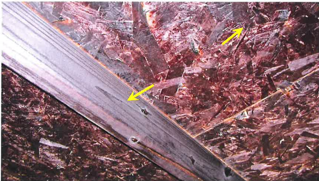
Photograph 28) – Close-up view of the fire-related effects from smoke on the pre-engineered wood truss and OSB sheathing.
