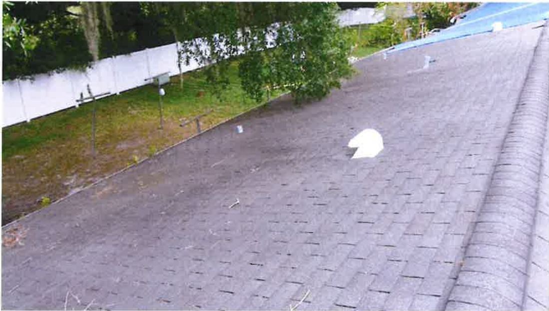
Photograph 19) – Roof overview looking northeast at the field zone of the west slope of the roof above Unit #19.
