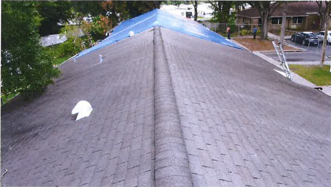
Photograph 15) – Roof overview looking north along the ridge of the roof above Unit #19 and #20.
