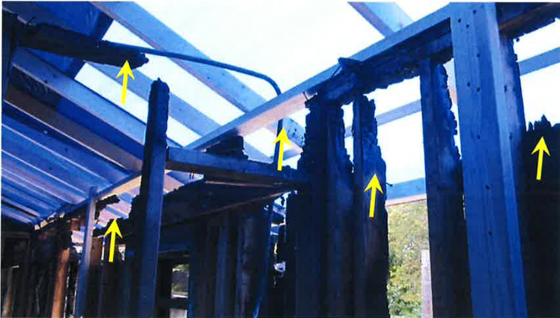
Photograph 43) – Interior view looking southwest at interior partition wall (left) and the rear exterior load-bearing wall of Unit #21. Arrows indicate upper portion of rear load-bearing wall framing system and interior partition requiring replacement.
