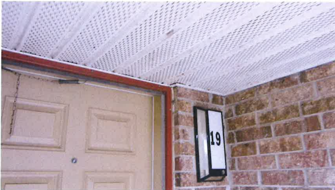
Photograph 7) – Close-up view of the exterior of Unit #19 at the front entry foyer.
