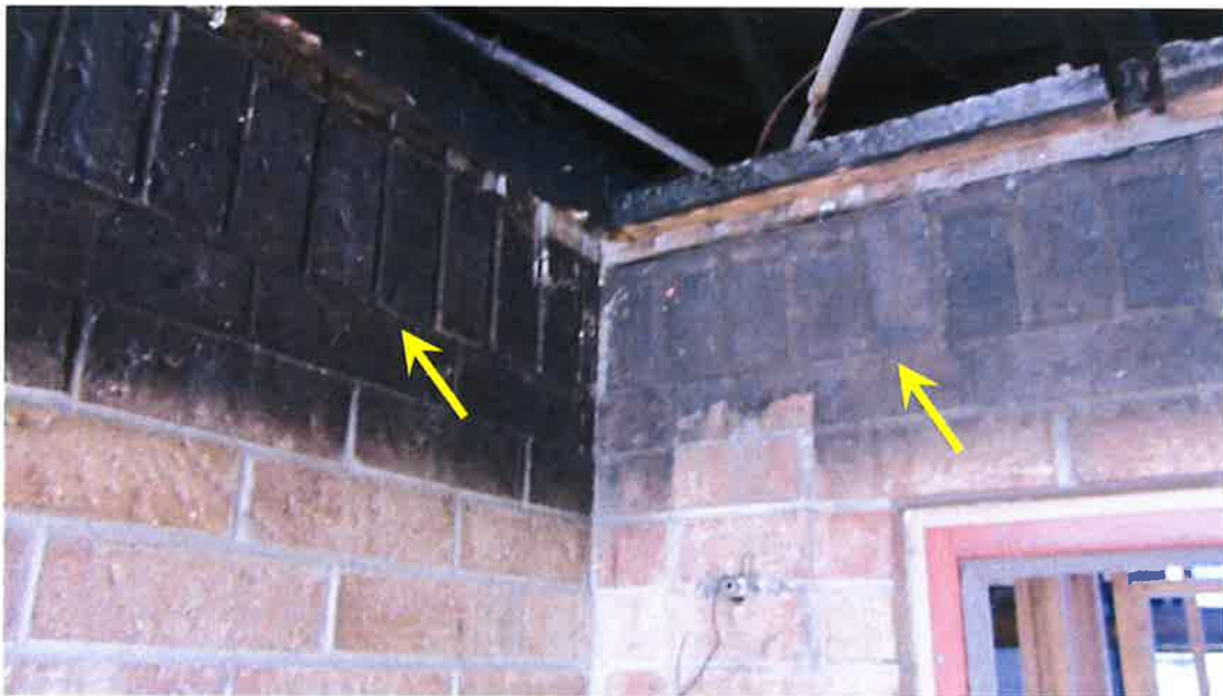
Photograph 58) – Close-up view of the exterior brick cladding at the front entry foyer of Unit #21. Fire-related effects from smoke shown with arrows.
