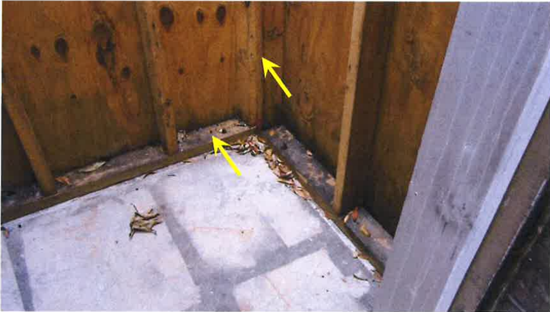
Photograph 55) – View looking at the exterior utility closet at the rear of Unit #22. Arrows indicate the lower portion of the wall framing system with no fire-related effects or damage.
