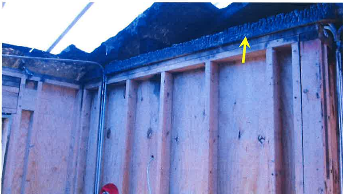
Photograph 44) – Interior view of exterior load-bearing walls at the front of Unit #21. Arrow indicates roof truss requiring replacement.
