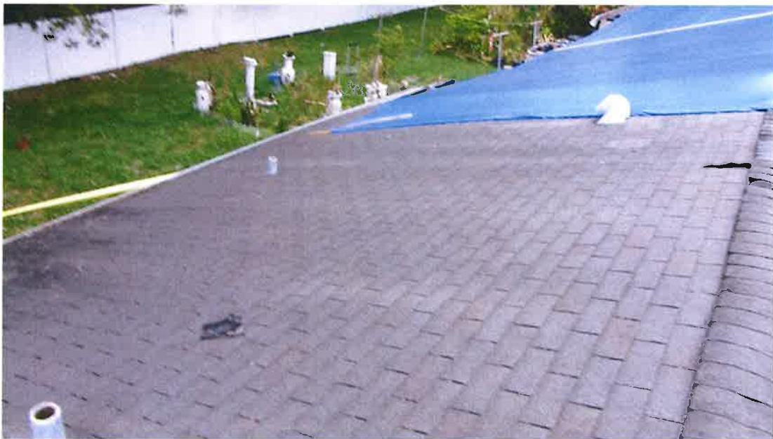
Photograph 22) – Roof overview looking northeast at the field zone of the west slope of the roof above the southern portion of Unit #20.
