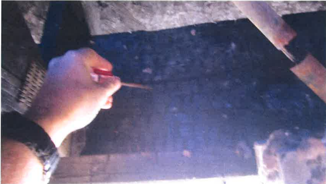
Photograph 37) – Close-up view of the west face of the double 2x12 wood header beam at the front entry foyer of Unit #20 requiring repair.
