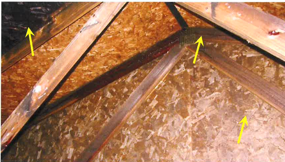
Photograph 24) – View looking south in the attic space above the southern portion of Unit #20. Right arrow indicates the separation wall between Unit #19. Middle and left arrows indicate fire-related effects from smoke.
