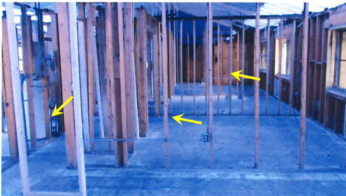
Photograph 48) – View looking north at the lower portion of interior partition walls in Units #21 and #22. No repairs required.
