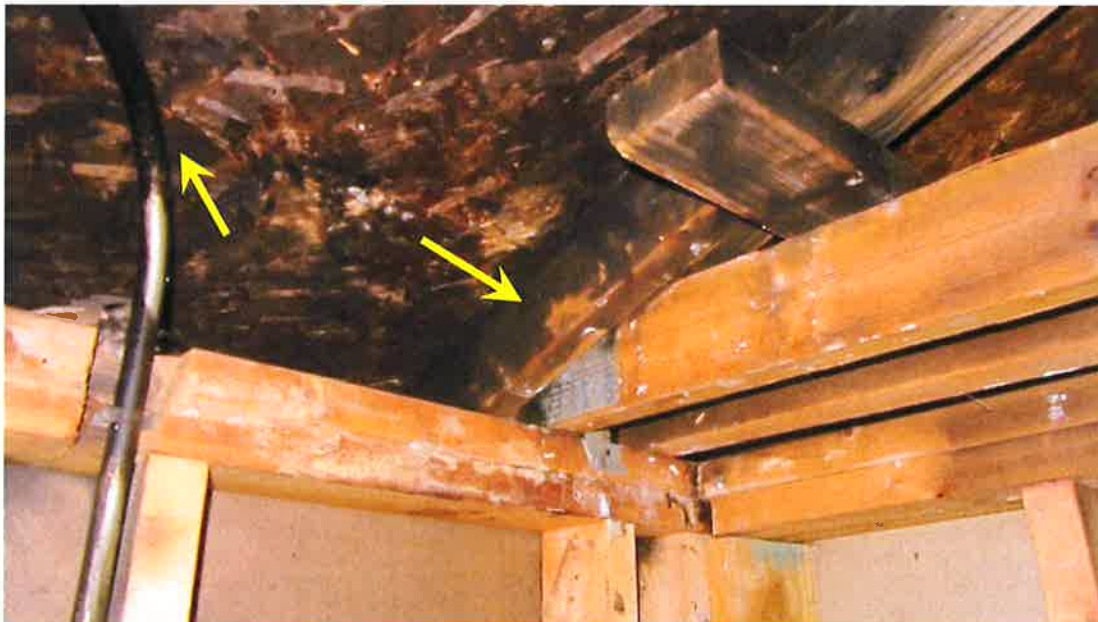
Photograph 30) – View of the east end of Truss 2 at the southern portion of Unit #20 and the connection to the top plate of the exterior wall. Arrows indicate fire-related effects from smoke.
