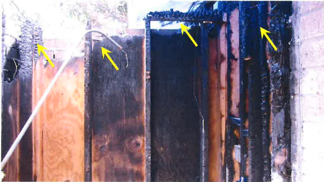
Photograph 49) – View looking north at the exterior utility closet at the rear of Unit #21. Arrows indicate fire-related damage to the upper portion of the wall framing system requiring replacement.
