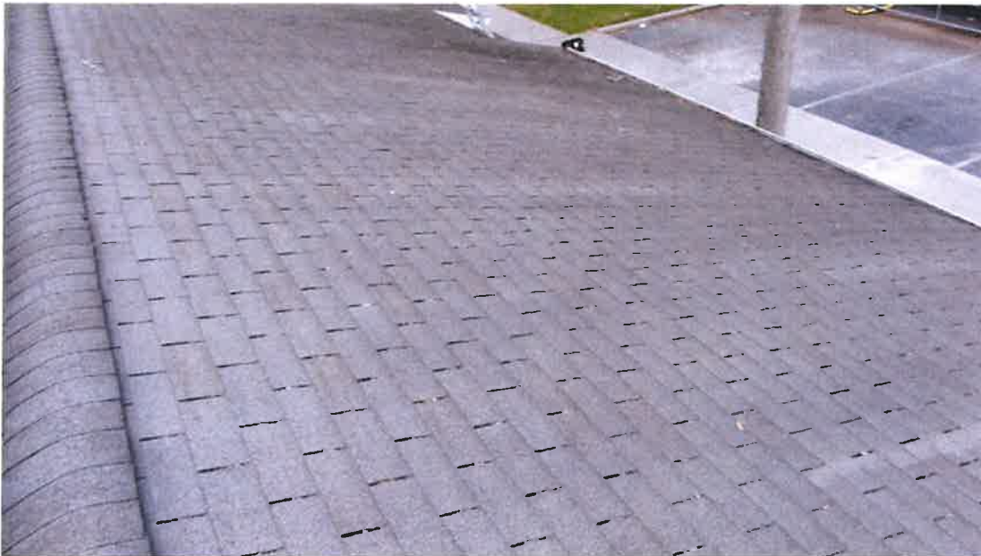
Photograph 17) – Roof overview looking northeast at the field zone of the east slope of the roof above Unit #19.
