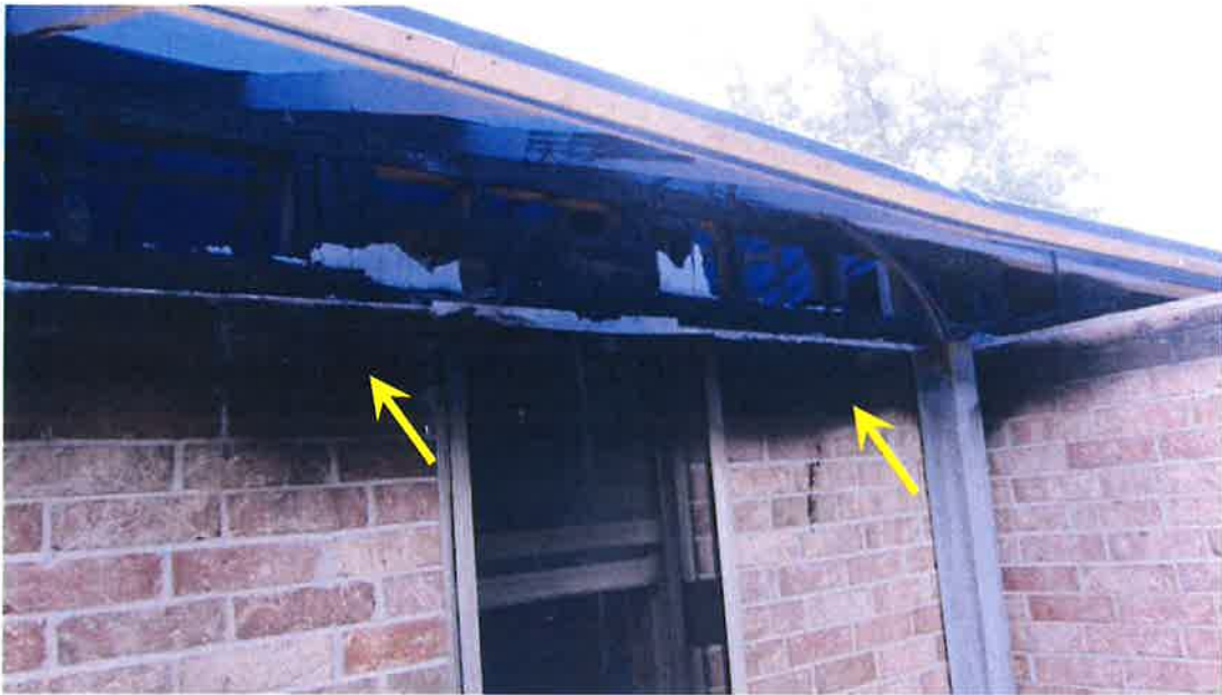
Photograph 63) – View of the exterior brick cladding at the rear of Unit #22. Fire-related effects from smoke shown with arrows.
