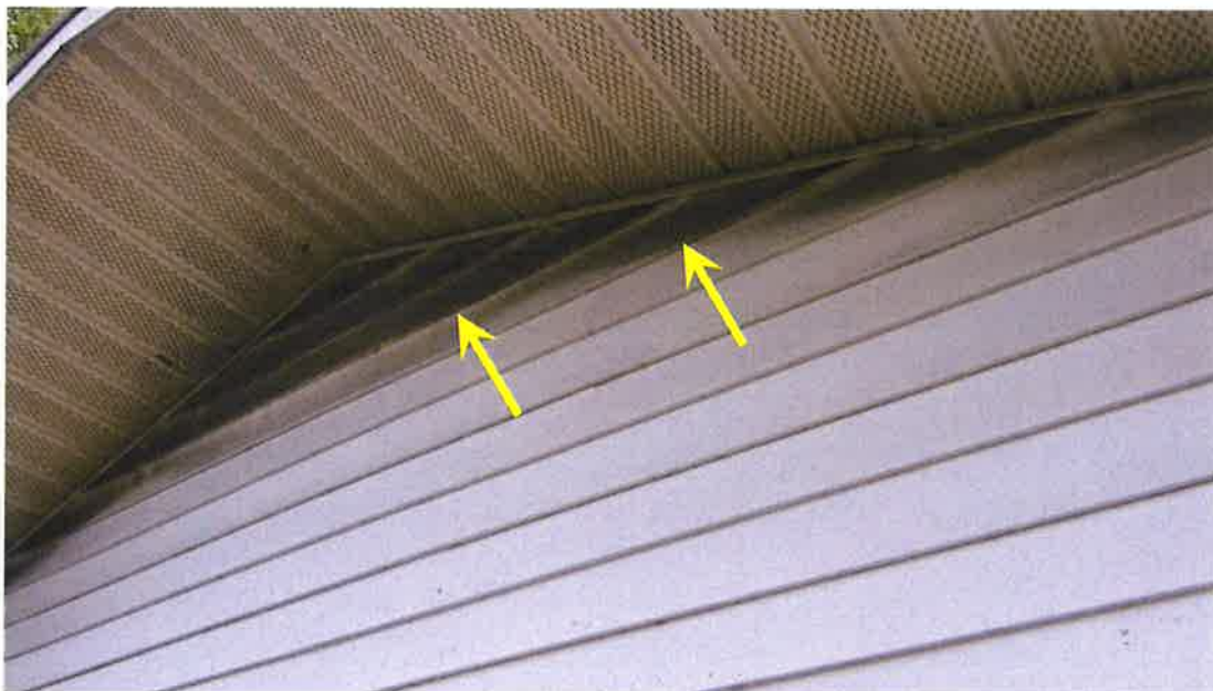
Photograph 8) – Close-up view of the soffit overhang and gable end siding at the south end of Unit #19. Arrows indicate fire-related effects from smoke.
