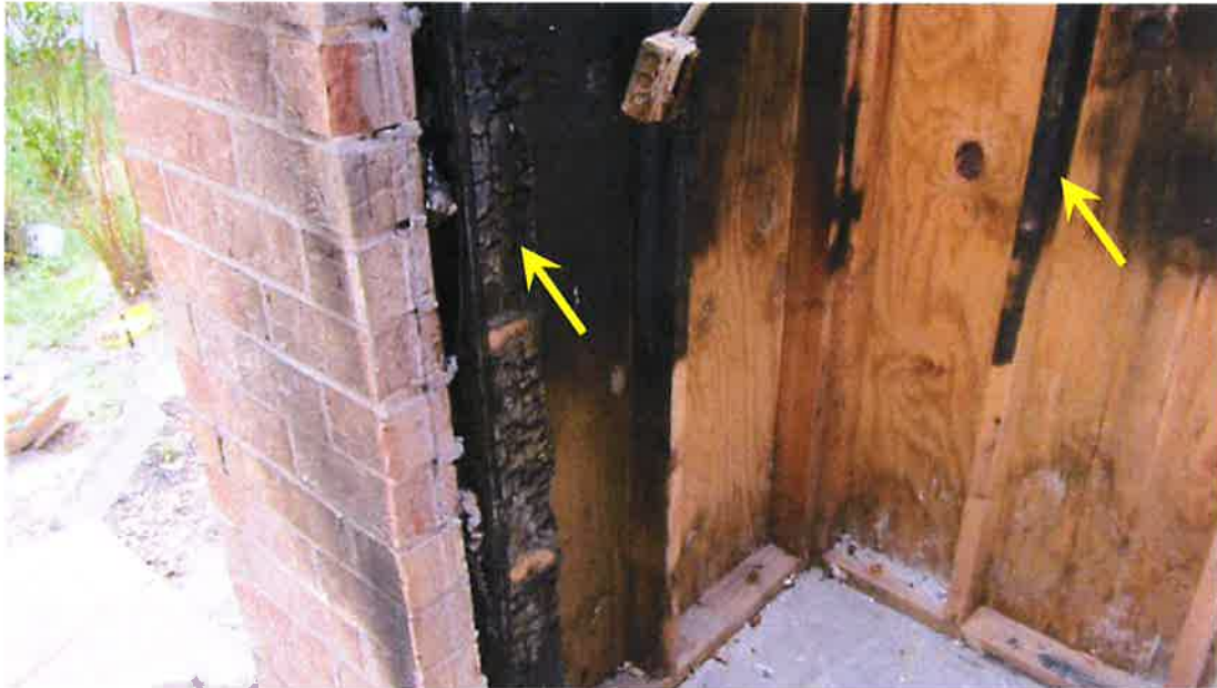
Photograph 51) – View looking northwest at the exterior utility closet at the rear of Unit #21. Arrows indicate fire-related damage to the upper portion of the wall framing system requiring replacement.
