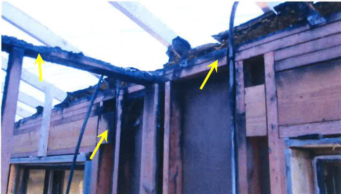
Photograph 41) – Interior view looking southwest at interior partition wall and the rear exterior load-bearing wall at Unit #22. Top left arrow indicates damage to the top plate of the partition wall requiring replacement. Remaining arrows indicate fire-related effects from smoke.
