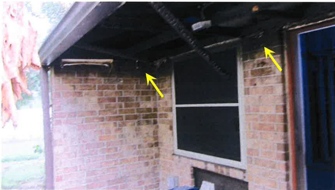
Photograph 64) – View of the exterior brick cladding at the rear of Unit #22. Fire-related effects from smoke shown with arrows.
