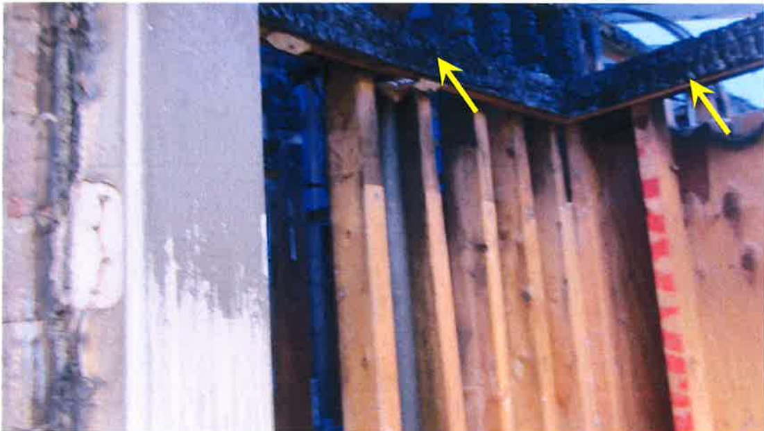
Photograph 54) – View looking southeast at the exterior utility closet at the rear of Unit #22. Arrows indicate fire-related damage to the upper portion of the wall framing system requiring replacement.
