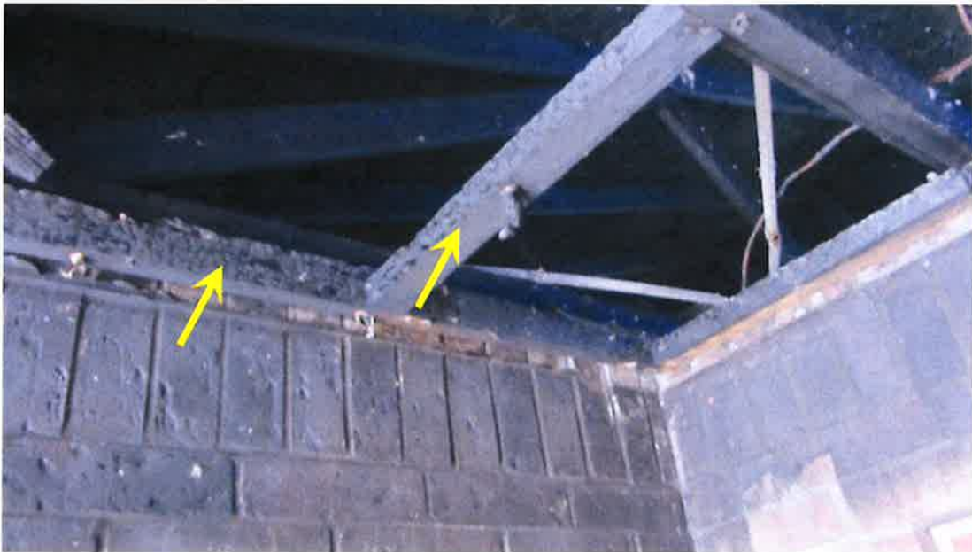
Photograph 33) – Close-up view the upper exterior wall at the front entry foyer of Unit #20. Arrow indicates fire-related damage to the wood ceiling framing.
