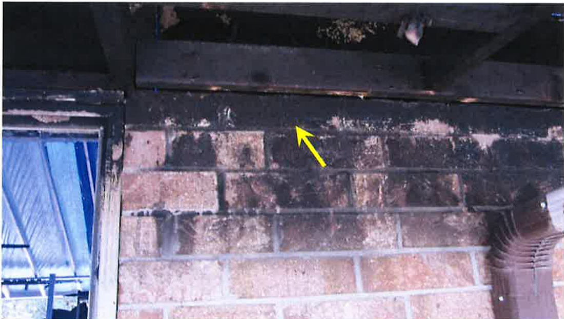
Photograph 59) – View of the exterior brick cladding at the rear exterior wall of Unit #21. Fire-related effects from smoke shown with arrows.
