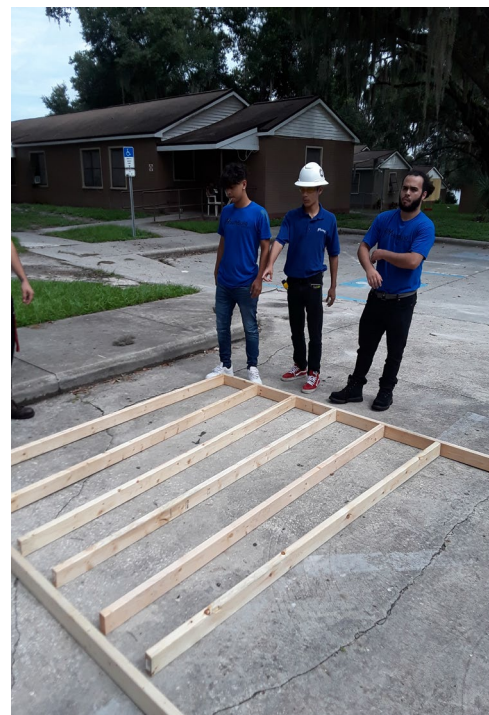
Left to right: Leonel Ortega , Wesley Santiago and Jose' Rivera are learning the skill of wall-framing at Twin Lakes.
