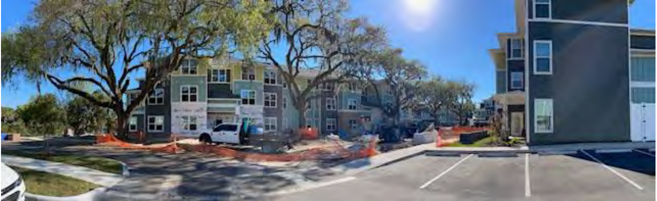
View of construction activity from parking lot south of the community center.
