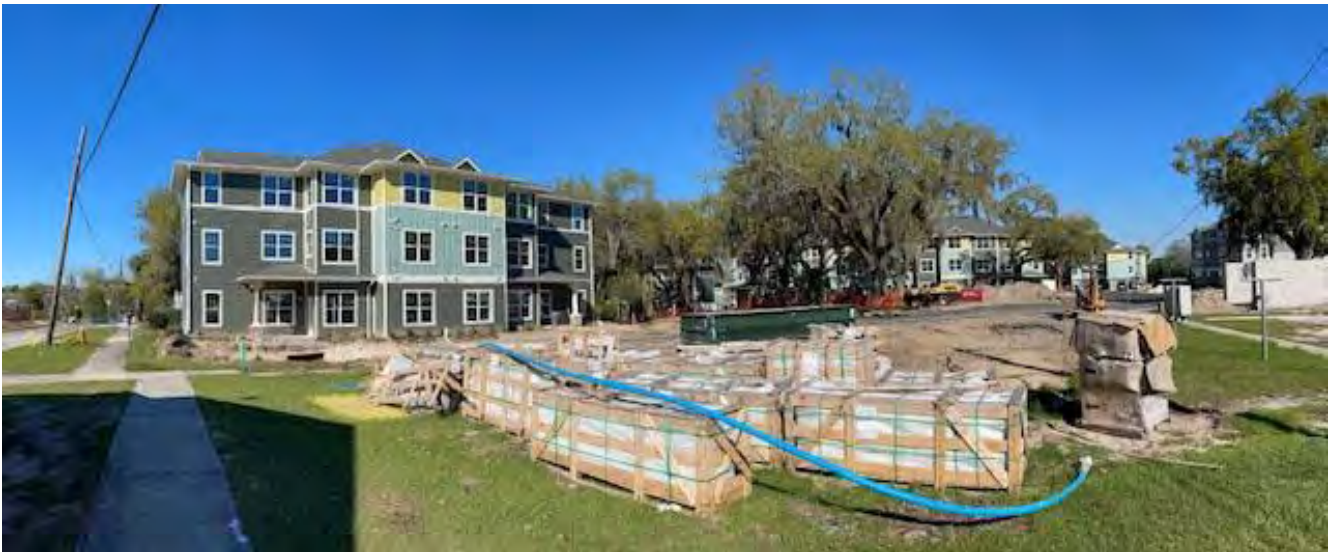
View of housing unit construction on the southwest side of the property.
