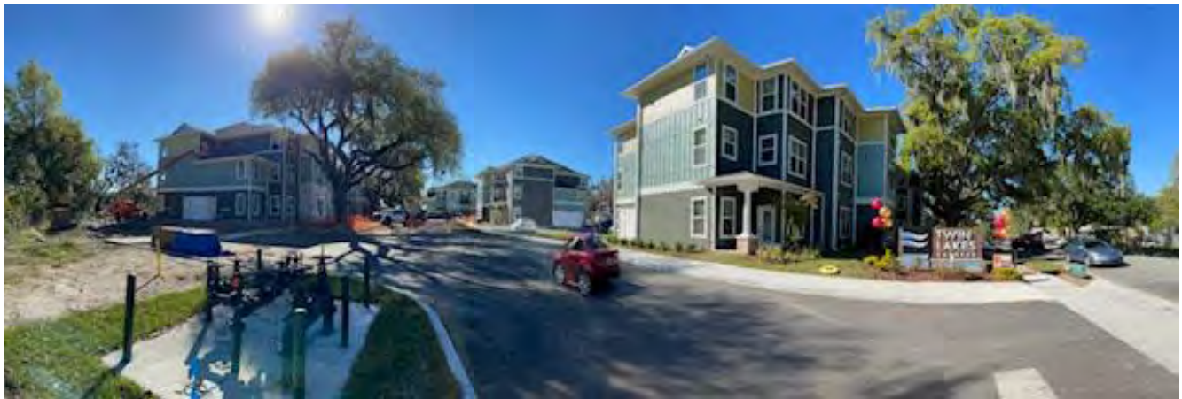
View of housing unit construction on the southeast side of the property.
