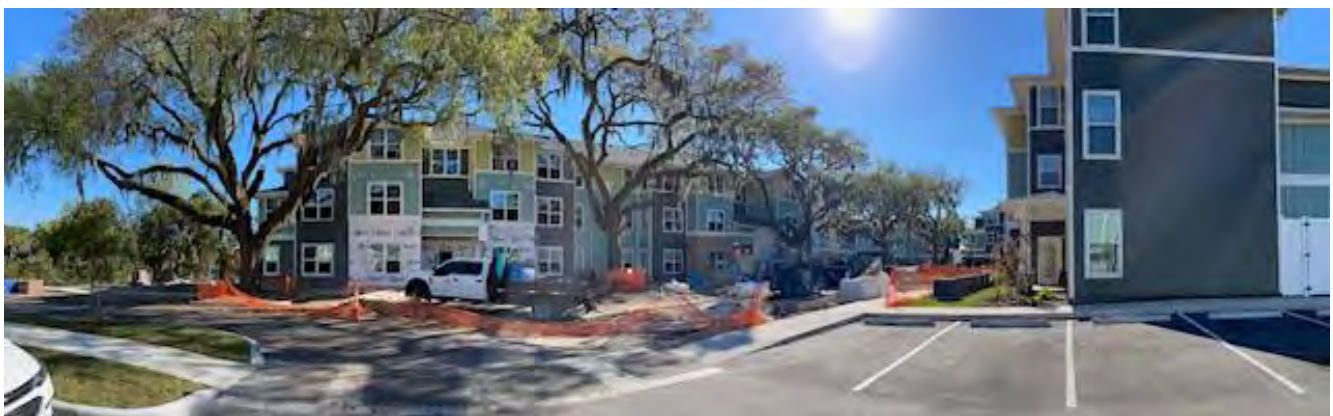
View of construction activity from parking lot south of the community center.
