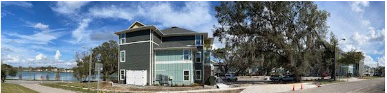
View of lake and housing unit construction on west side of property.
