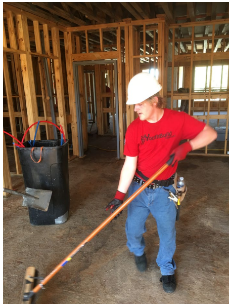
Wesley Soles, YBL participant busy on the construction site at Twin Lakes.
